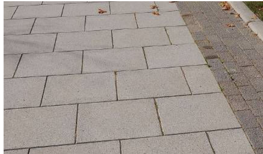
Concrete slabs used on a pavement in a Feature Square at Jennett's Park
